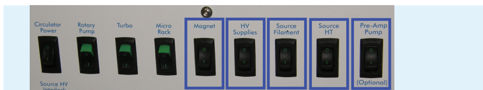
Figure 2.5-4: Switches in the off position.
