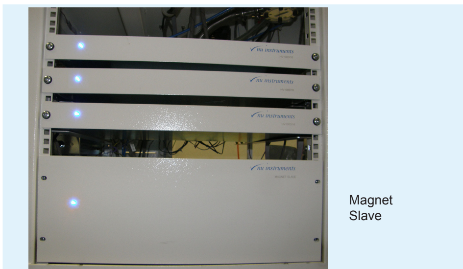
Figure 1.8-7: Magnet Slave and HV1000/16 units.
