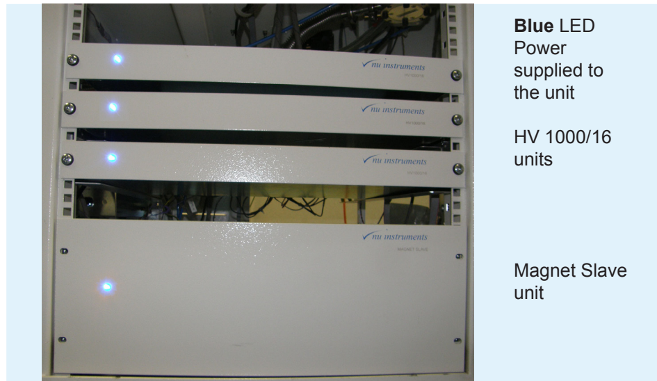
Figure 1.8-9: HV1000/16 units and Magnet Slave units.
