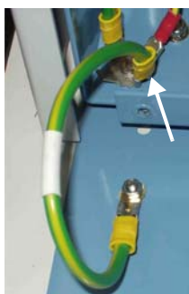
Figure 3-38. Grounding cable of right side panel
