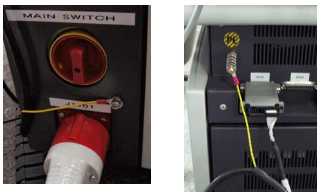
Figure 8-9. Grounding cable at MAT 253 (left) and DELTA series (right)
